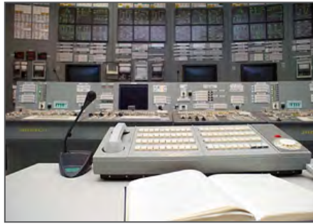
Programmable logic control systems
