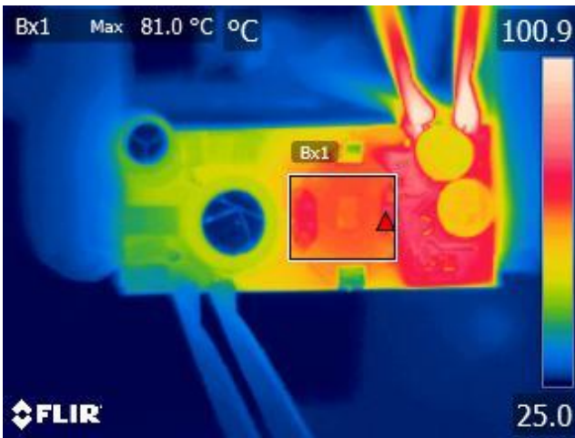
Figure 42 – Ambient = 25 °C. Transformer, T2 = 81 °C.
