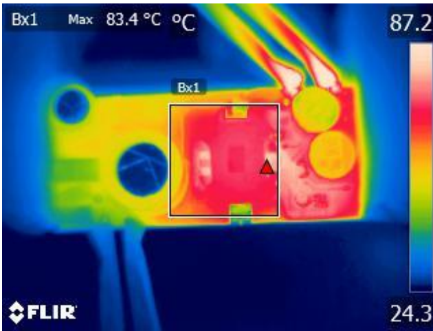
Figure 34 – Ambient = 24.3 °C. Transformer, T2 = 83.4 °C.
