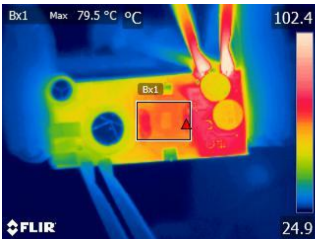
Figure 38 – Ambient = 24.9 °C. Transformer, T2 = 79.5 °C.
