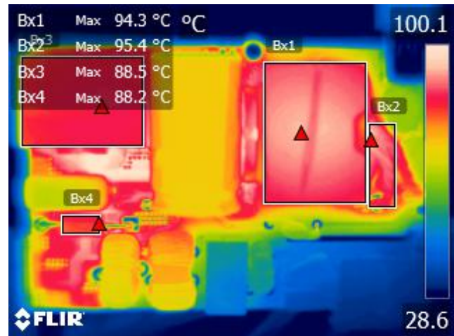
Figure 59 – Top Thermal Image, T_{AMB} = 27.9 °C. Bx1: Transformer Core = 94.3 °C. Bx2: Transformer Wire = 95.4 °C. Bx3: PFC Inductor Core = 88.5 °C. Bx4: Boost Pre-charge Diode = 88.2 °C.
